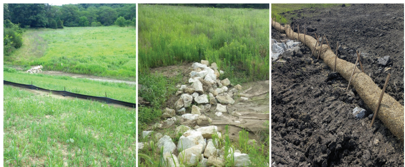
Examples of ESCDs: silt fence (left), check dam (middle), wattle (right)
