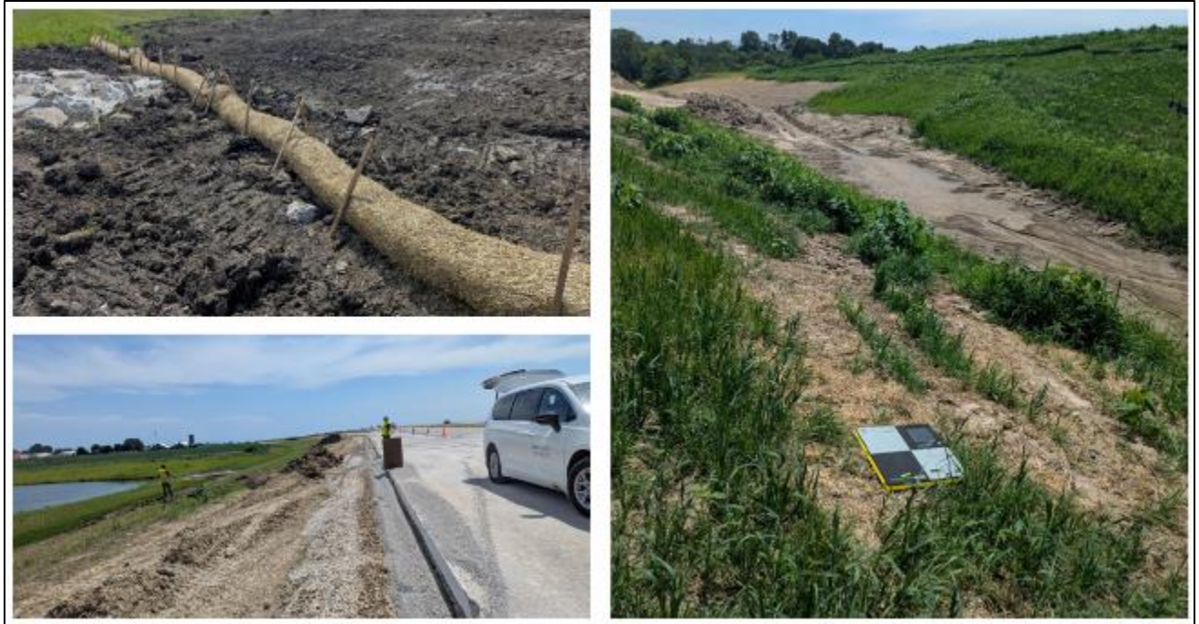
Figure 5. Erosion and sediment control devices at Mediapolis Site 2, including wattles, a reseeded slope, and a check dam
